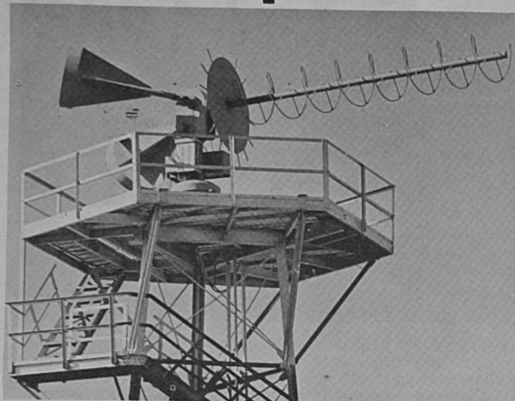
BEST ANGEL —This helical antenna has been positioned by 5th Weather Wing personnel so it can receive the best signals possible from the ESSA 6 weather satellite. Satellite signals are properly filtered to separate picture information from static interference. (Air Force photo)
